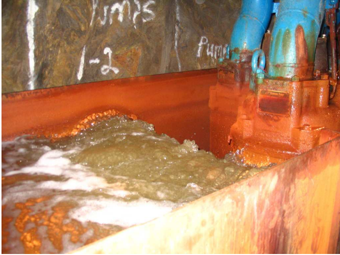
Pumps at 4100ft
