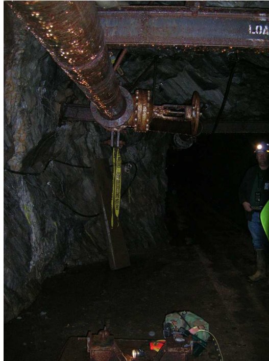
Humidity (now 300ft station)
