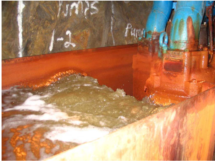
Pumps at 4100ft
