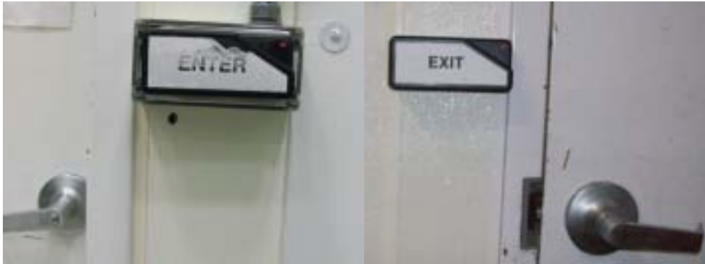
Figure 3: Entry and exit door swipes for the LVEA. On the right photo, a Kantech automated door striker is visible to the left of the door handle.
