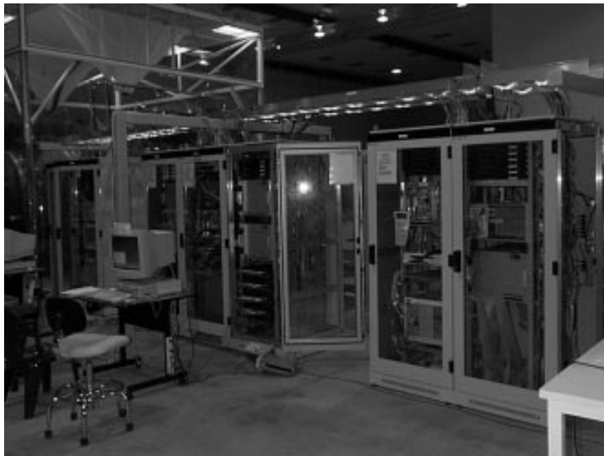
Control System Racks
