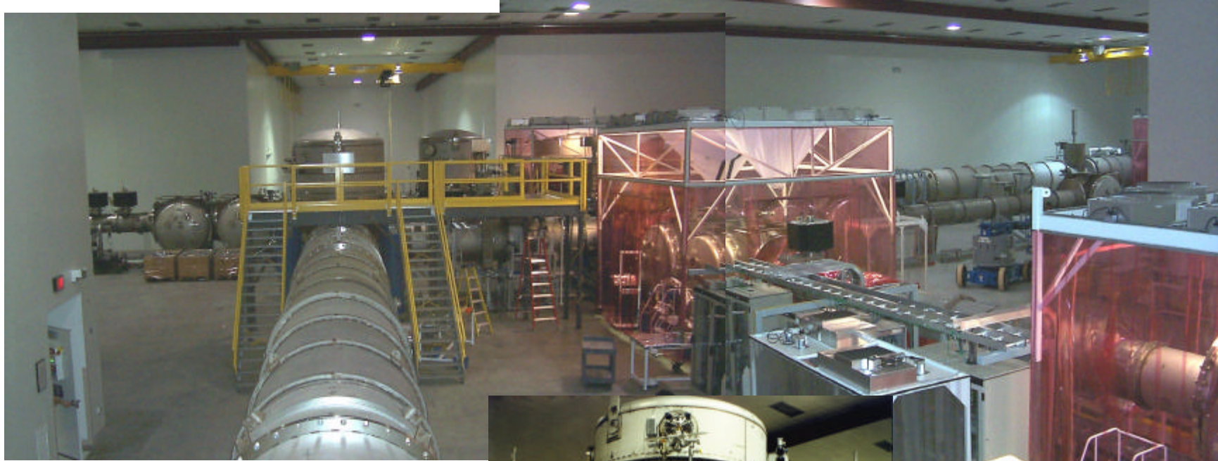
View inside Corner Station
