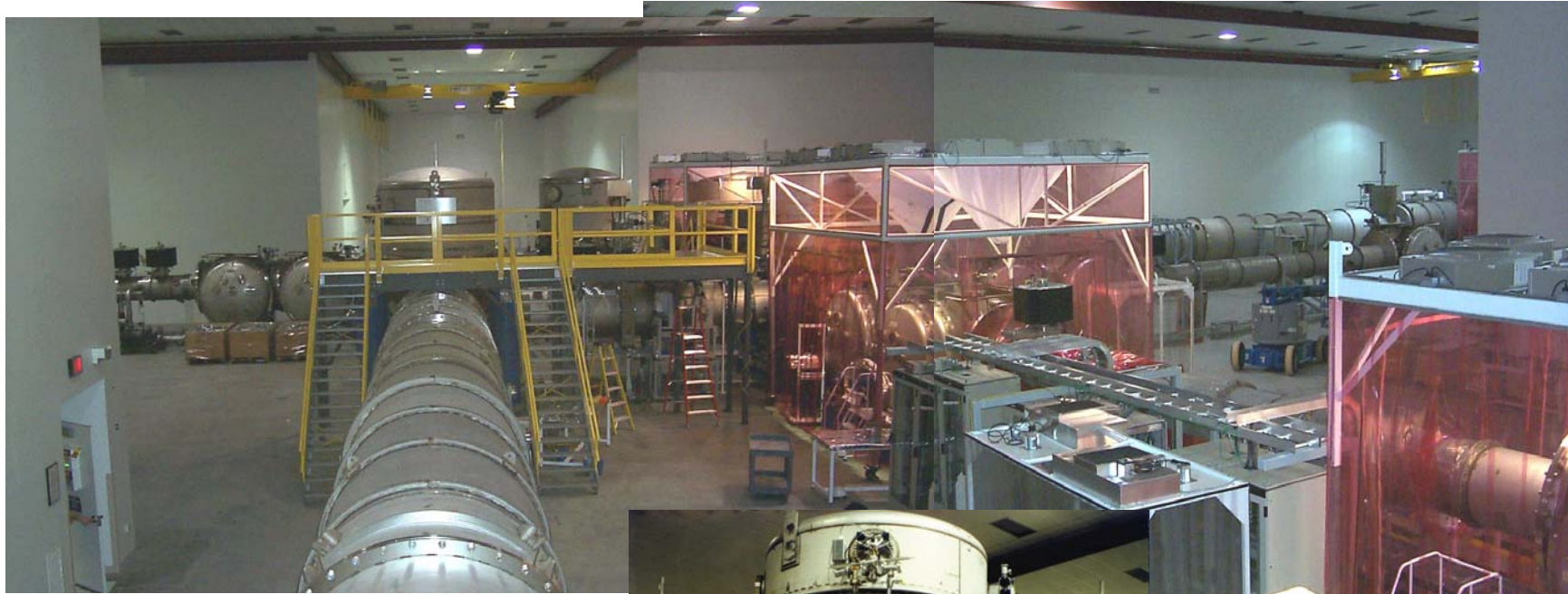
View inside Corner Station
