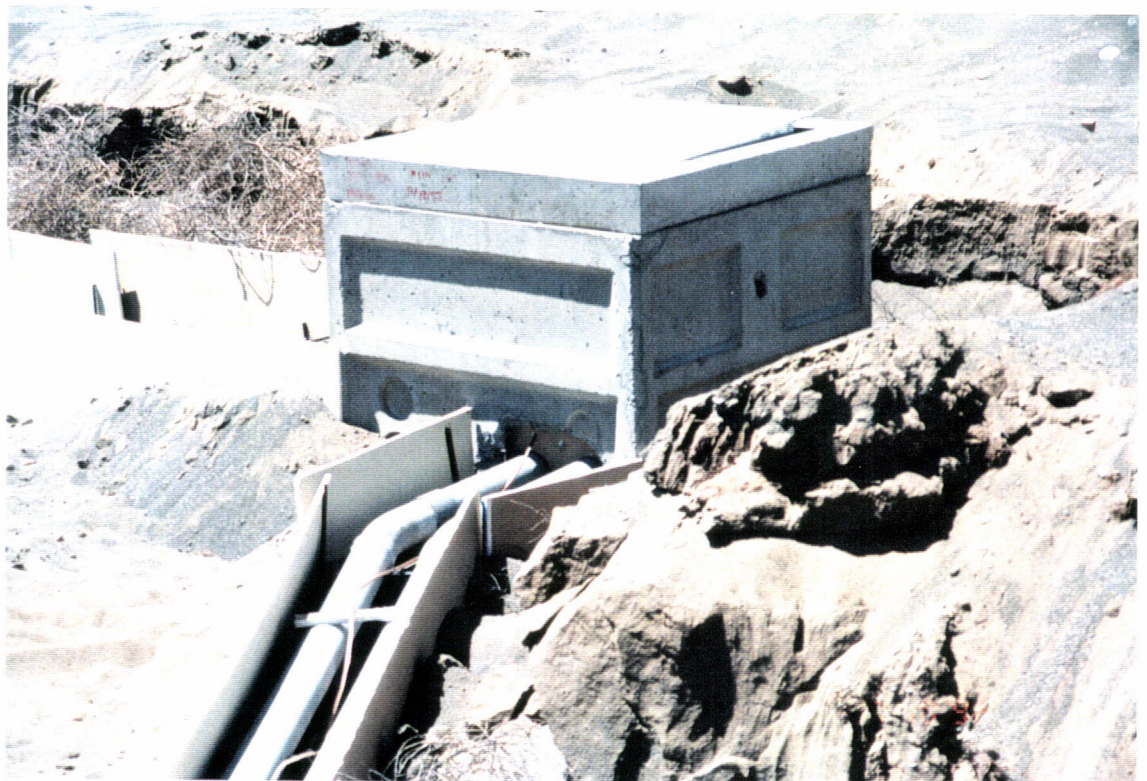
Typical duct bank for the supply power from the transformer to the electrical cable pull box.
