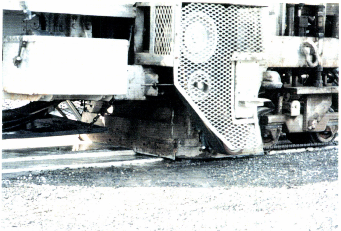
Close up view of the grinding equipment that is grinding the alignment groove in areas where the elevation of the alignment groove is out of specification.
