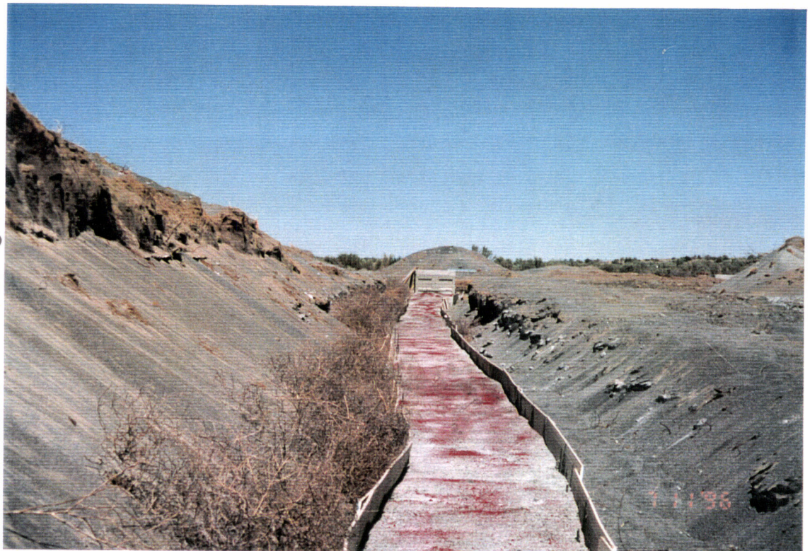
Red oxide is scattered on top of duct bank prior to concrete curing.
