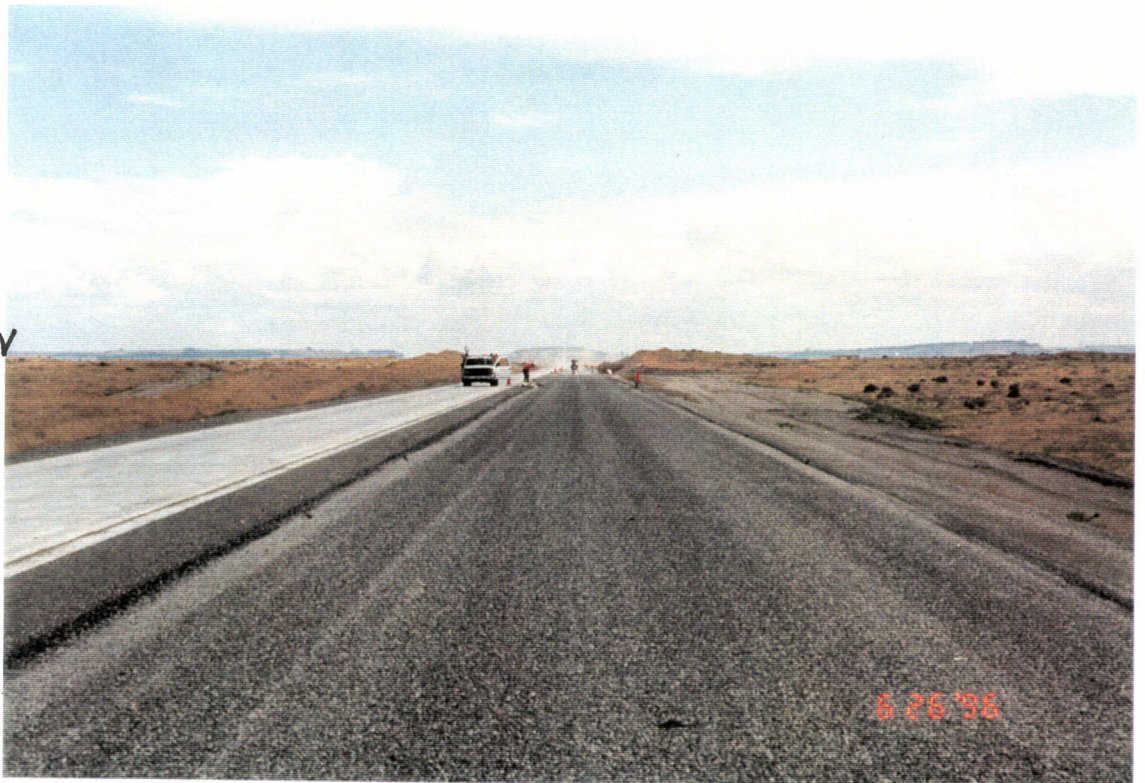
View of the northwest arm where the road surfacing is virtually completed.
