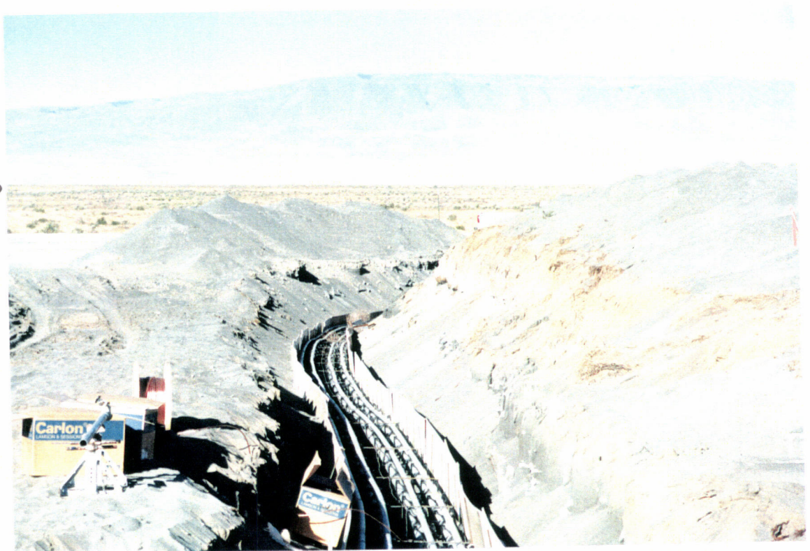
View of the conduit for the duct bank at the northwest arm End Station.
