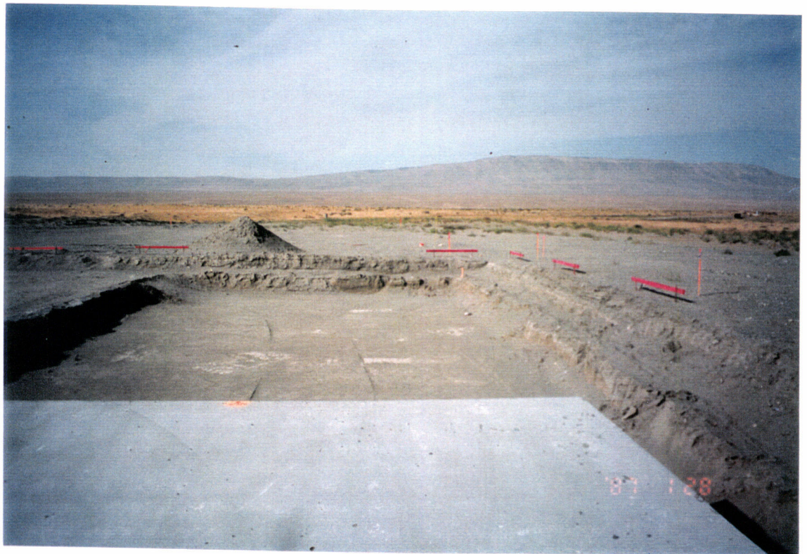
32- Different view from the end of the slab, of the SW arm end station.
