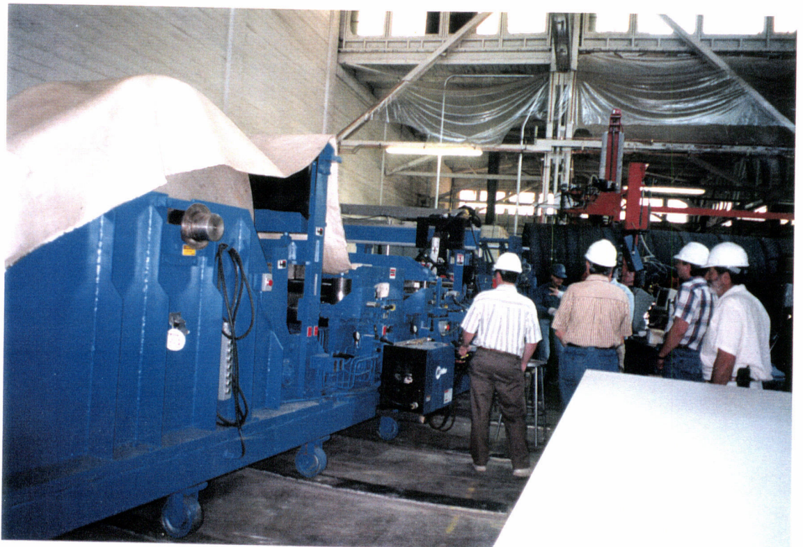
42- Spiral tube mill - on the coil feed side.
