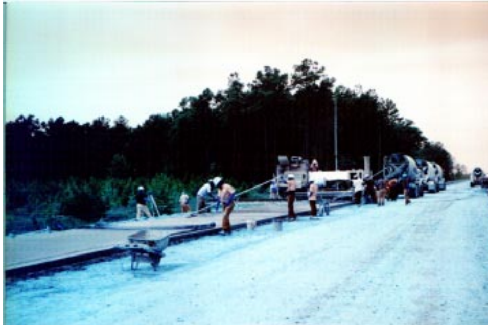
Figure 11. Placing Concrete for the Beam Tube Enclosure Slab along the 'X' (Southwest) Arm at the Livingston Site.
