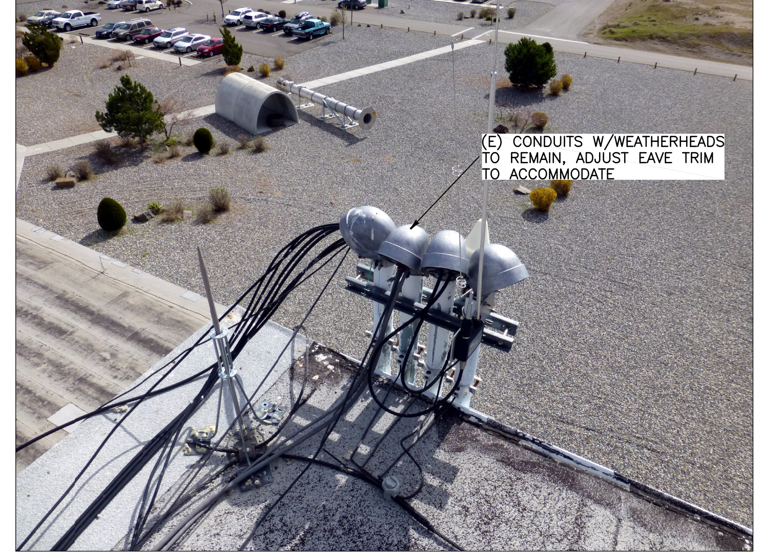
PHOTO 10 WEATHERHEADS CONDITION REF
