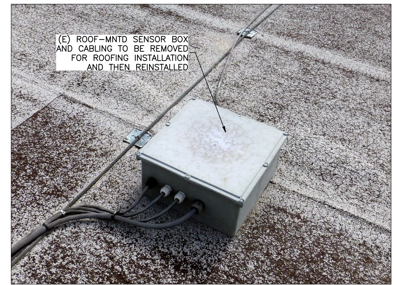
PHOTO 11 (E) SENSOR BOX AND CABLING CONDITION
