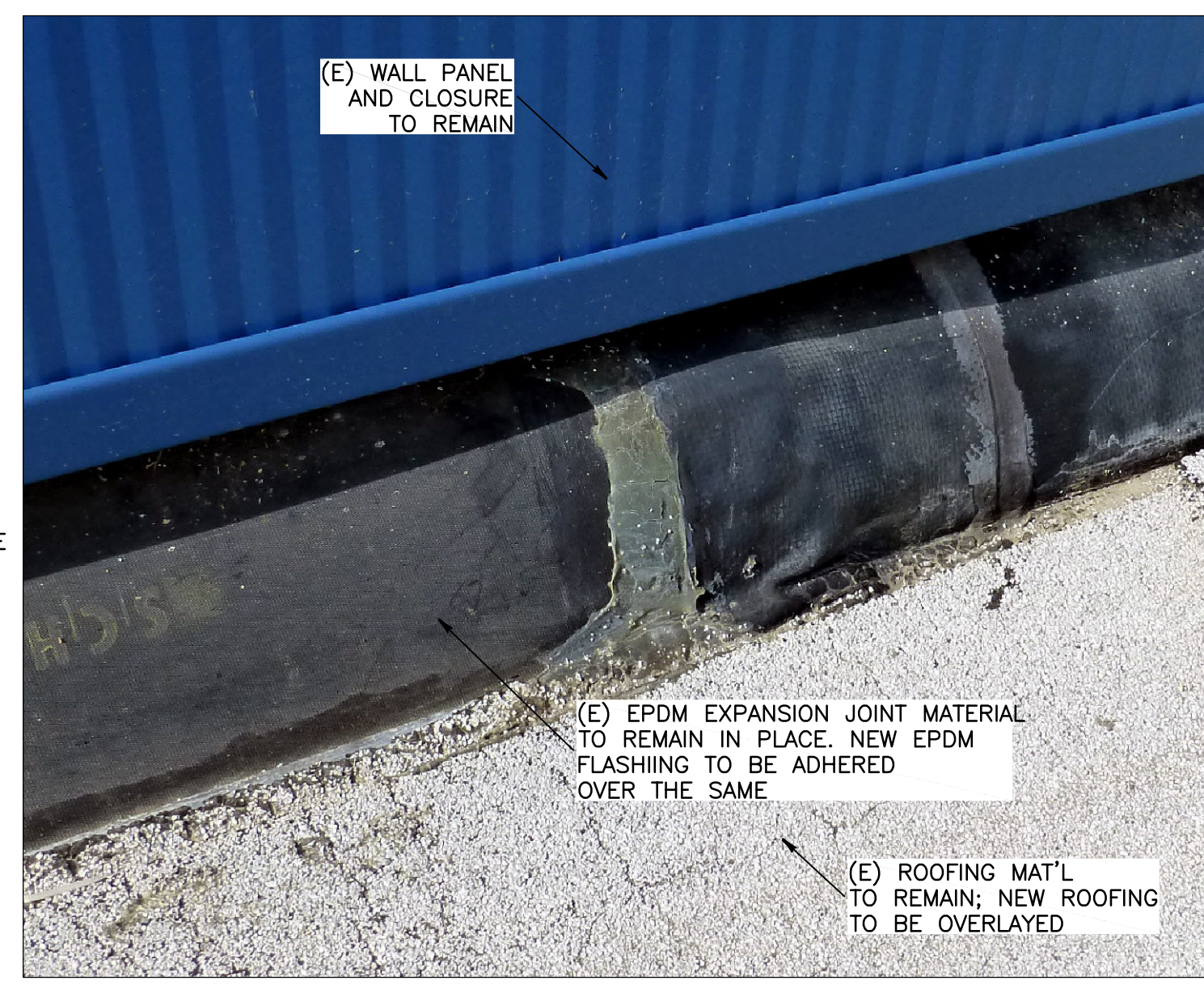
PHOTO 2 EXISTING EXPANSION JOINT CONDITION REF
