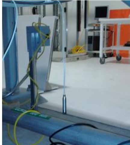
Figure 3: An Installed Microphone
