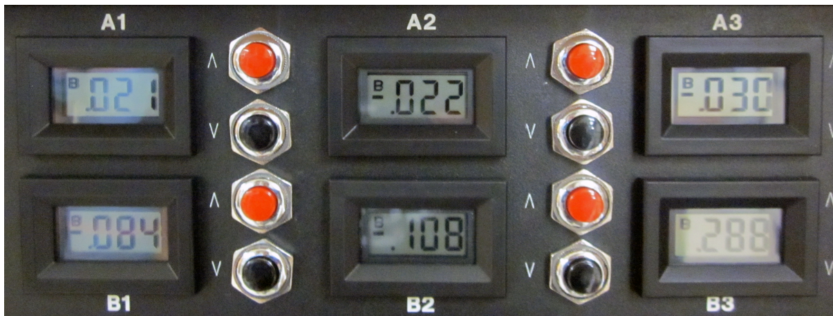
Figure 4: The DC motors box with the readouts for the voltage offset (in mV). From left to right, the top readouts correspond to the top motors (TS—top- south—, TW, TE) and the bottom ones to the bottom ones (BN, BS, BE). The red buttons are used to extend the motors and the black ones to shorten them.
